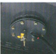
Maintenance hole for cleaning
